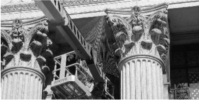
Bird control netting being installed at the U.S. Post Office building in NYC.
