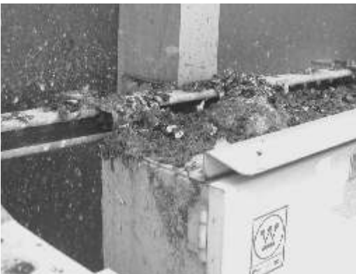
This electrical box is a fire waiting to happen.
