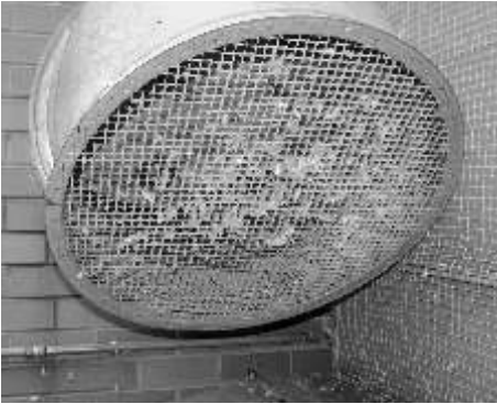
Buildings and inhabitants are at risk when dried feces can infiltrate a building through the air handling equipment.
