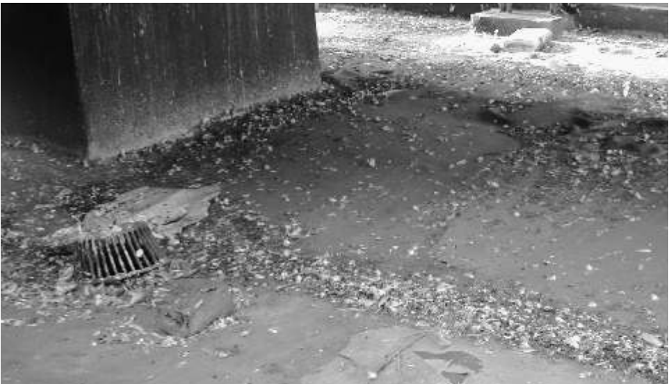
Bird droppings, feathers and nesting material clogged this drain causing extensive water damage and structural damage.
