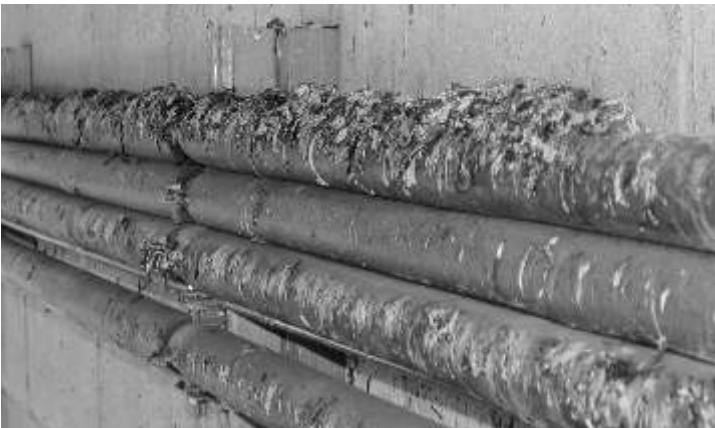
These pipes will soon be spouting leaks. The corrosion caused by bird droppings can eat right through metal and paint.
