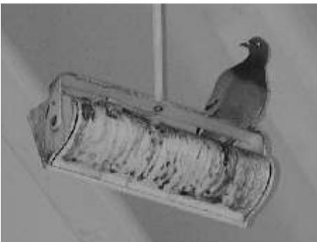
Metal and paint are susceptible to corrosion from bird droppings.
