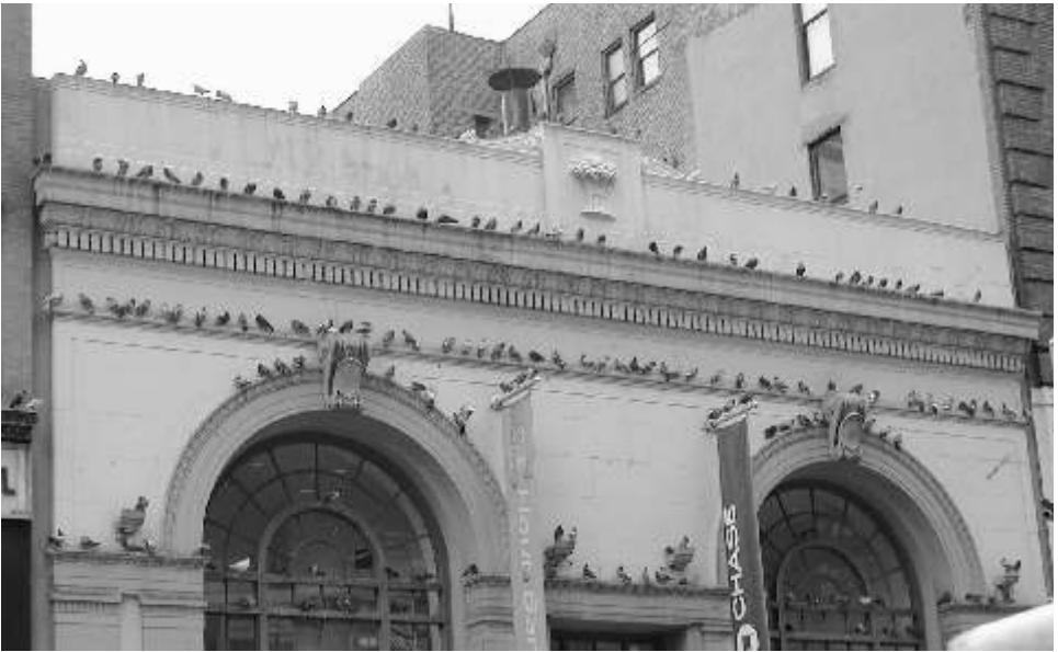
Unfortunately, this is all too common a scene on buildings without proper bird control.
