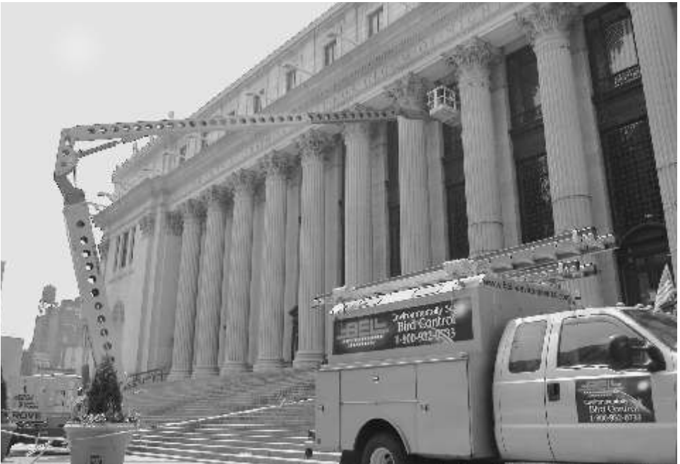
Even elaborate, historic buildings can be protected from the defacing that accompanies pest birds. Here, Bell Environmental Bird Specialists install bird control on the United States Post Office building in New York City.
