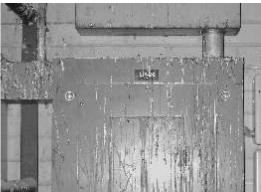
The next person to work on this electrical panel should wear rubber gloves and a approved face mask.
